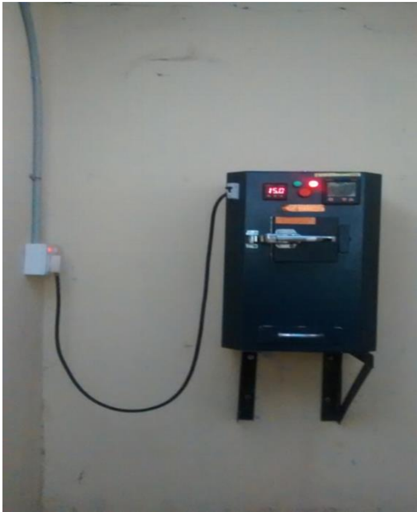
Napkin Vending Machine and Incinerator
