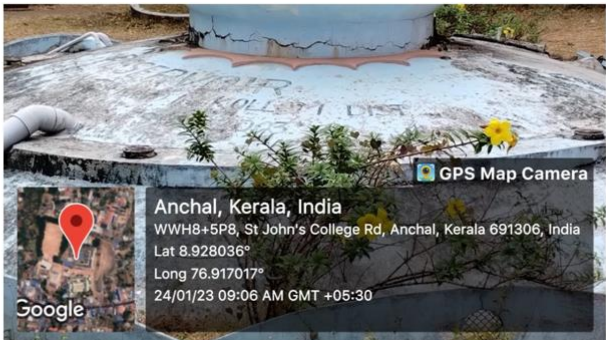
Water harvesting tank with capacity 1.5 lakh litres
