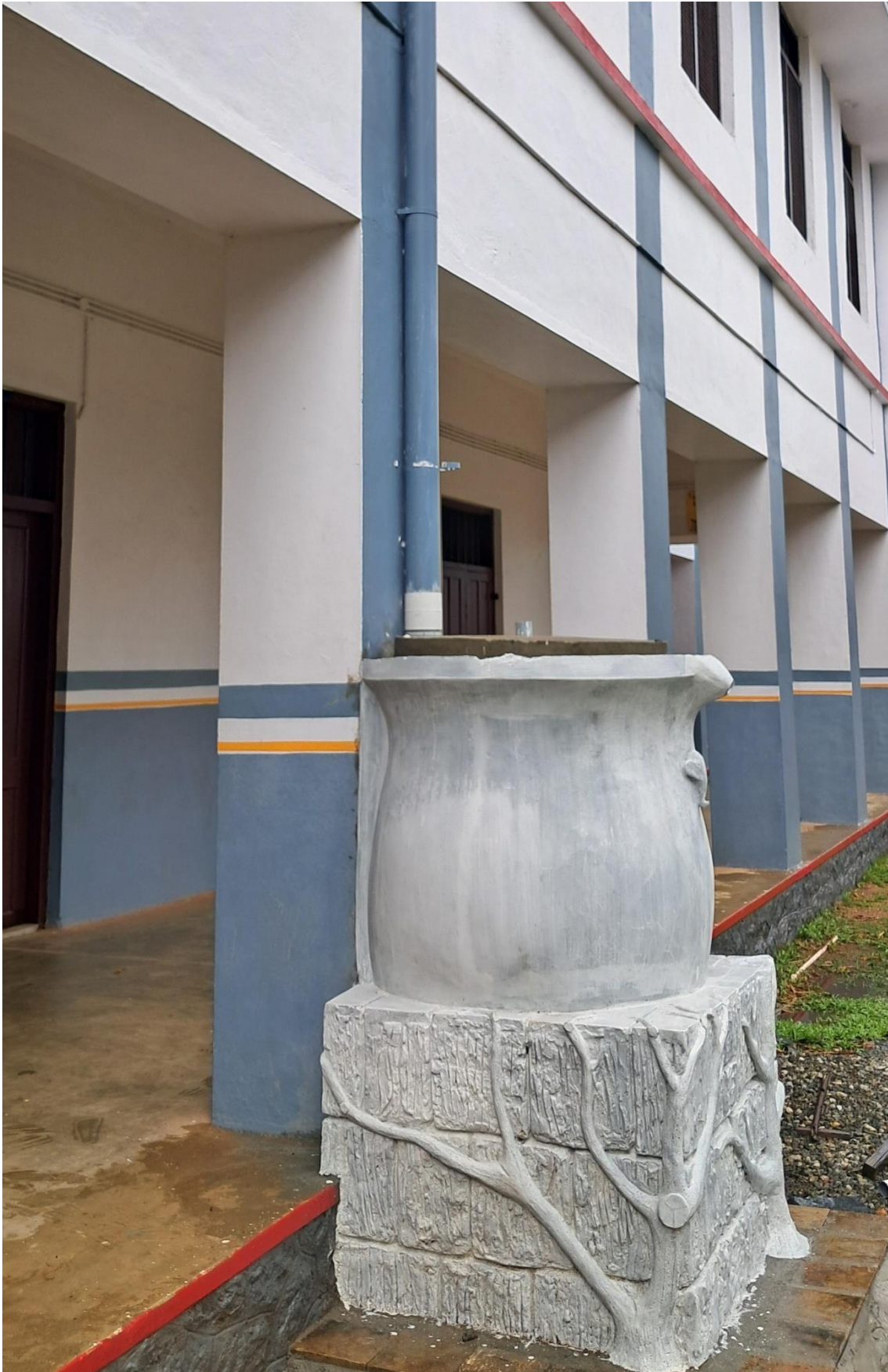
Unified water collecting pits for water harvesting from roof tops
