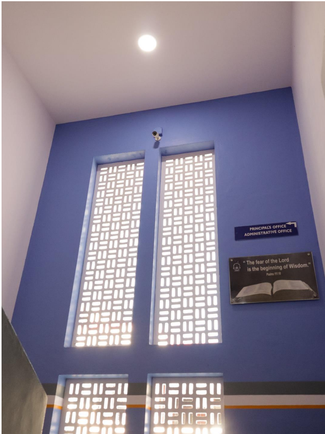
CCTV cameras at different locations inside the campus
